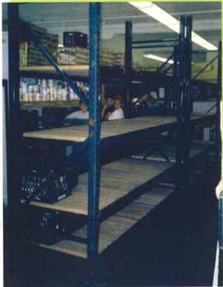
One of many shelves installed at the Issaquah Food Bank for my Eagle Scout Project
